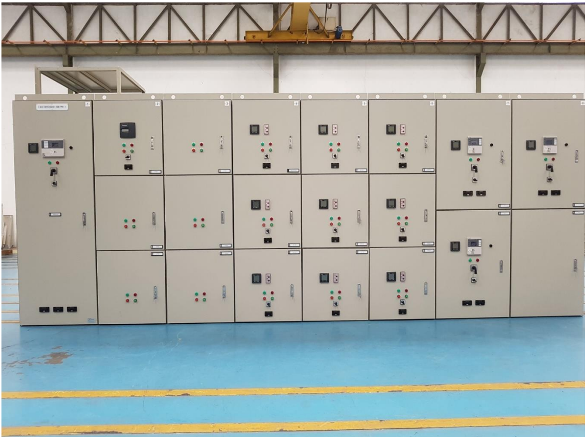
3.3kV Switchgears , Motor Control Center , Capacitor Bank
