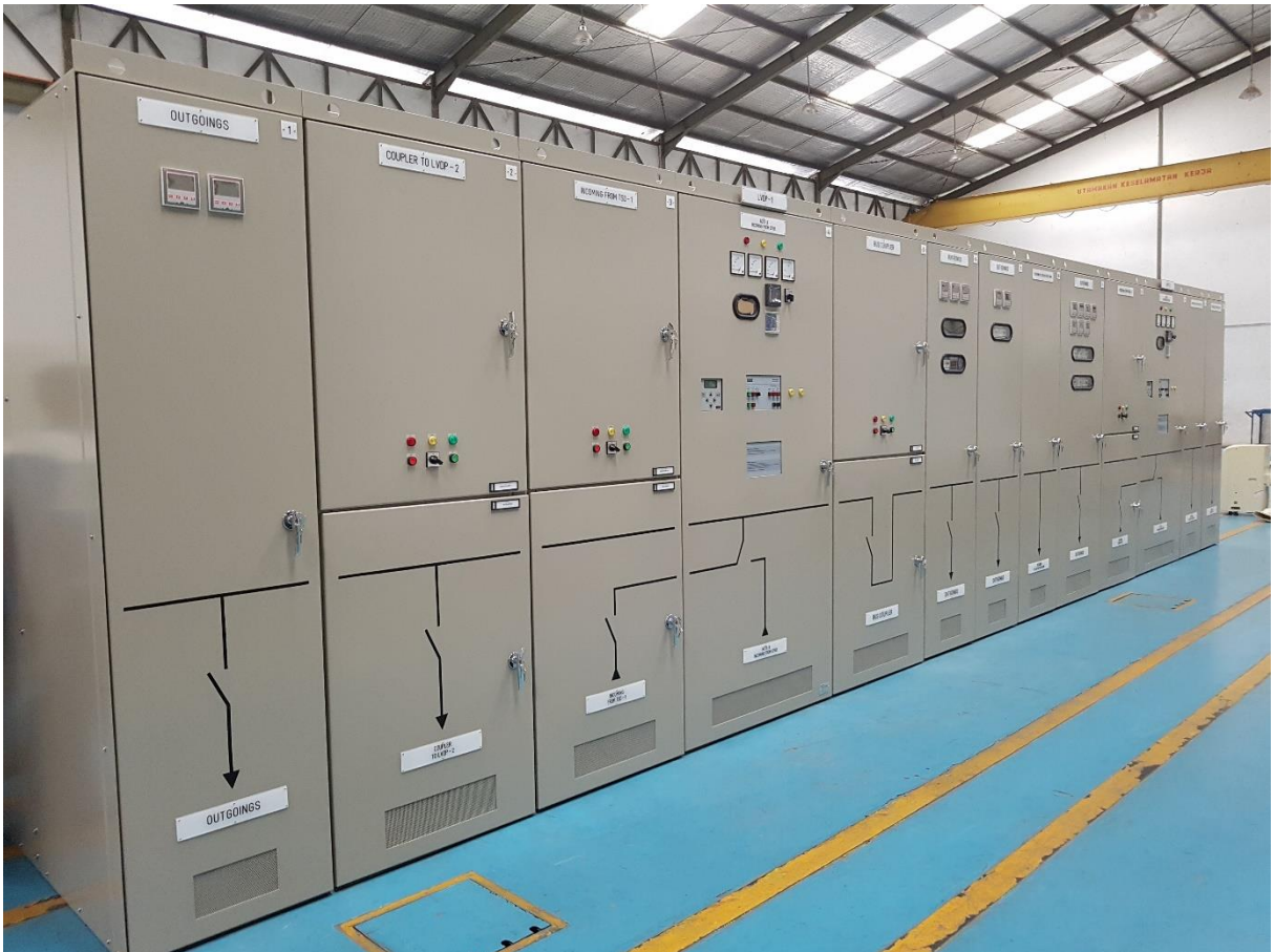
400V Switchgears , Auto Transfer Switch (ATS)
