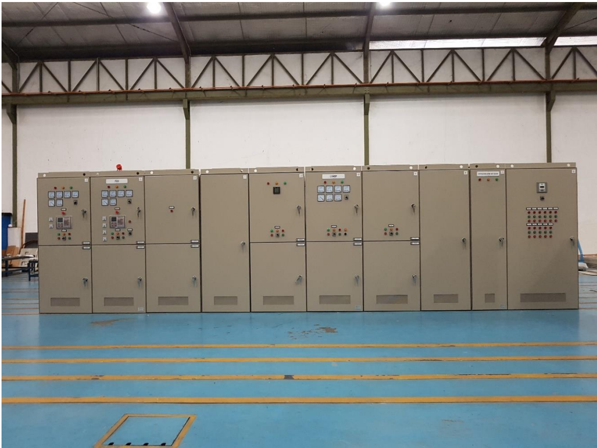
400V Switchgears , Auto Synchronizing Generator, Auto Transfer Switch (ATS) and Capacitor Bank
